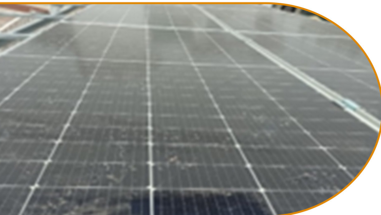
Solar Off Grid Installation
