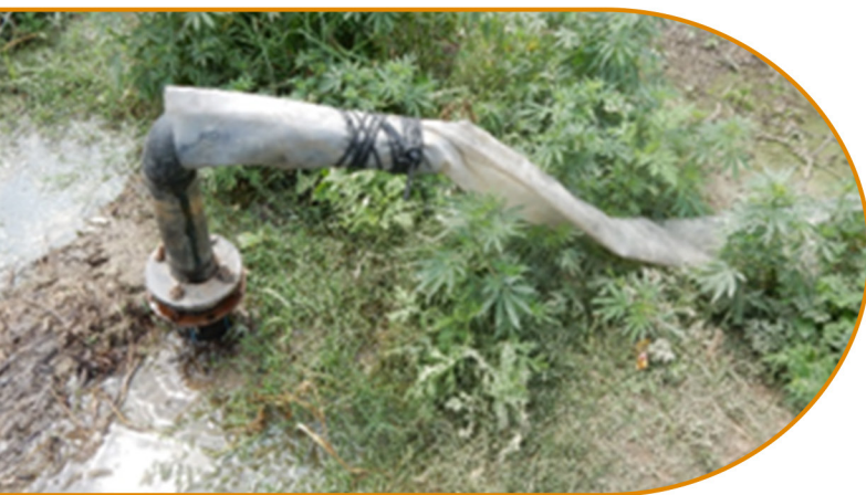
Pipeline for excess water supply for irrigation purpose
